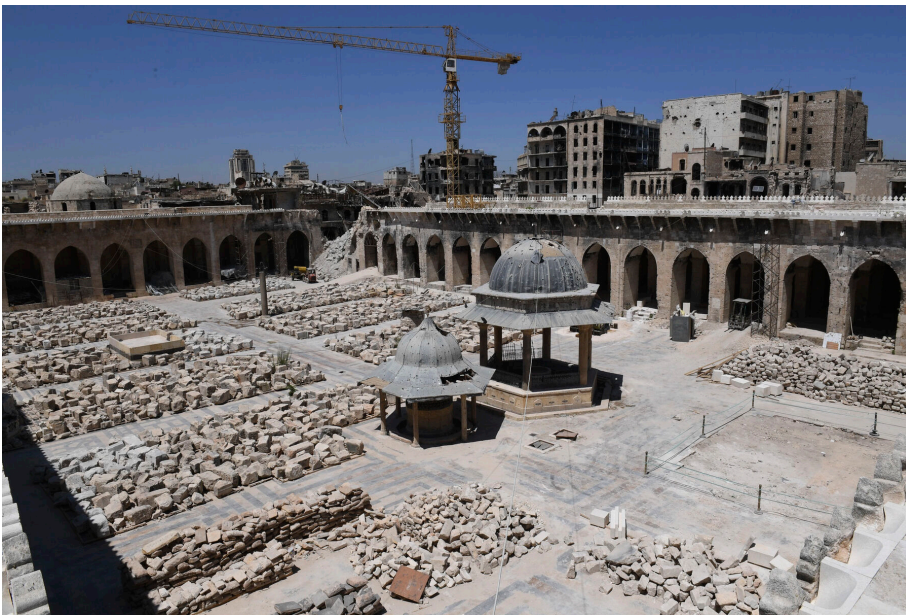
Figure 12.2 Restoration work underway at the Great Mosque, or Umayyad Mosque, in the Old City of Aleppo, 14 August 2018. A crane stands over the rubble of the toppled thirteenth-century minaret, whose stones have been catalogued and organized in the mosque’s courtyard. (Photo by George Ourfalian/AFP via Getty Images)
